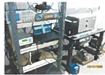
Ammonia sensor and electronics installed on Moody Tower roof.
